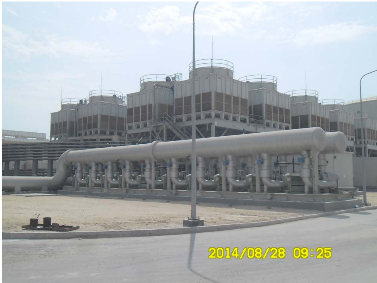
Figure 3 Secondary Chilled Water Pumps
