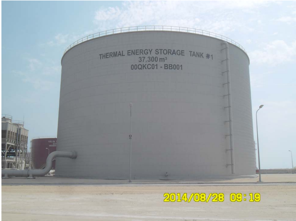
Figure 1 Thermal Energy Storage Tank
