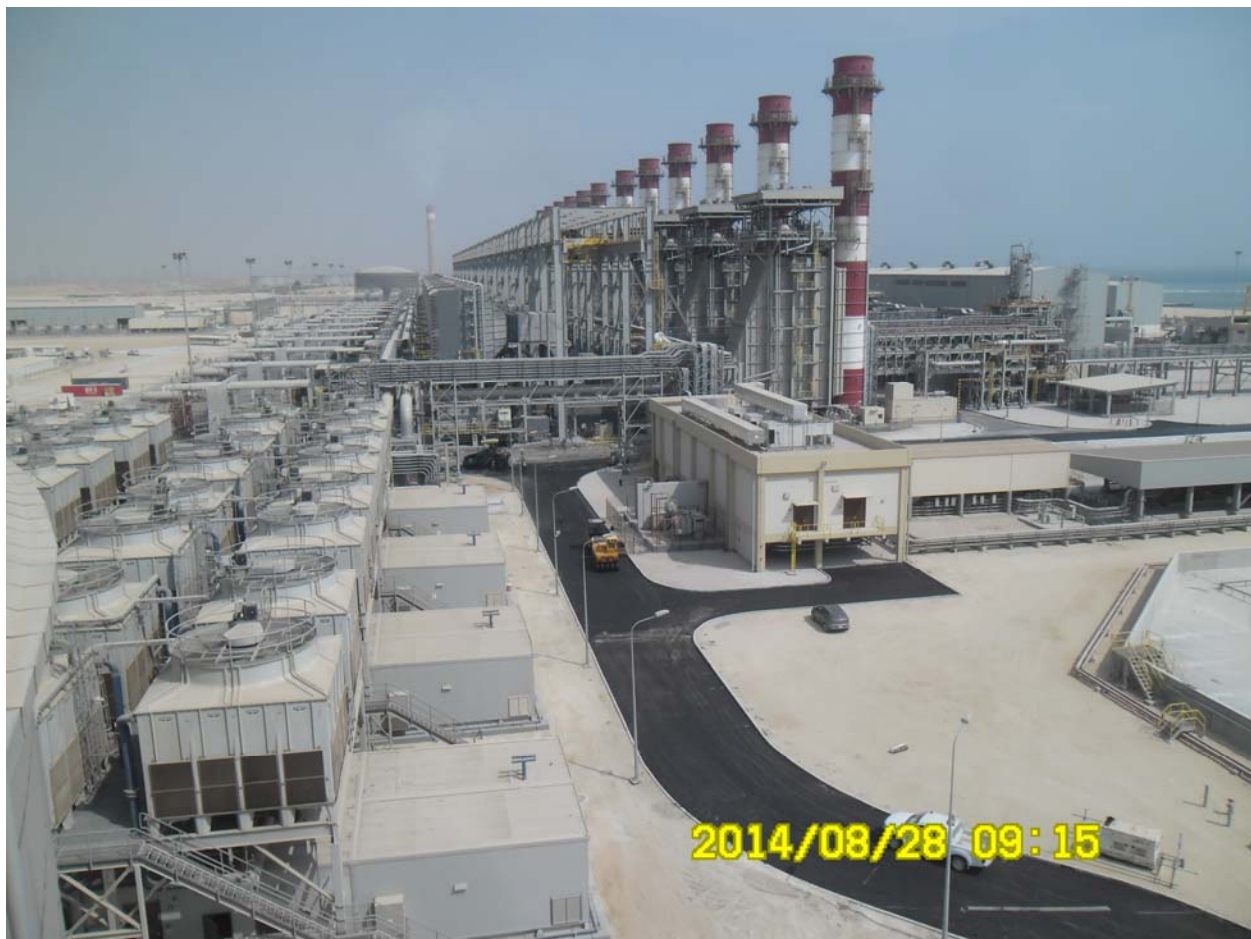
Figure 4 Power Block Overview
