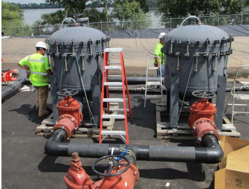
Figure 7: The two 100-micron bag filters of the temporary water treatment plant.
