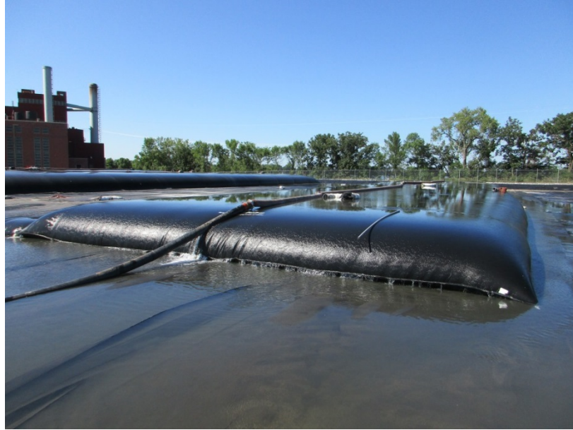
Figure 6: A geotextile dewatering tube being filled with the CCR and sediment slurry.
